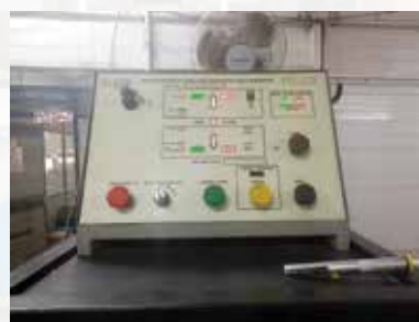
Station Master Panel
