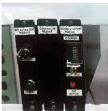
Station Master Panel
