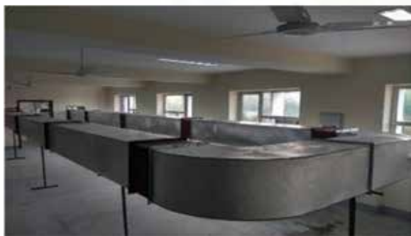
Fig: HVAC Ducting System a) Air Handling Unit and b) Duct system with integrated Disinfectant solutions
