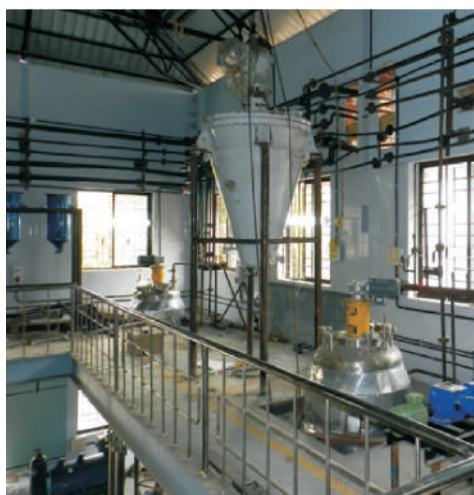
Fig. Pretreatment Reactor
