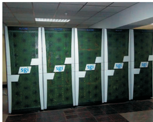
Fig. HPC system Altix ICE 8400
