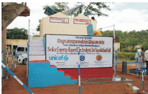
Fig. Solar power based EDF plant at the Adiwasi Kanya Shiksha Parisar, Chhindwara
