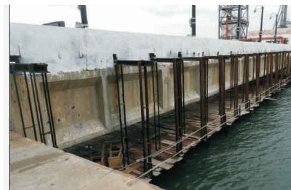
Fig. Investigated distressed PSC girder of span 3 of off-shore tanker terminal of VPT
