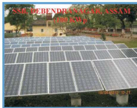
Few off-grids Power Plant installed at different location of SSB
