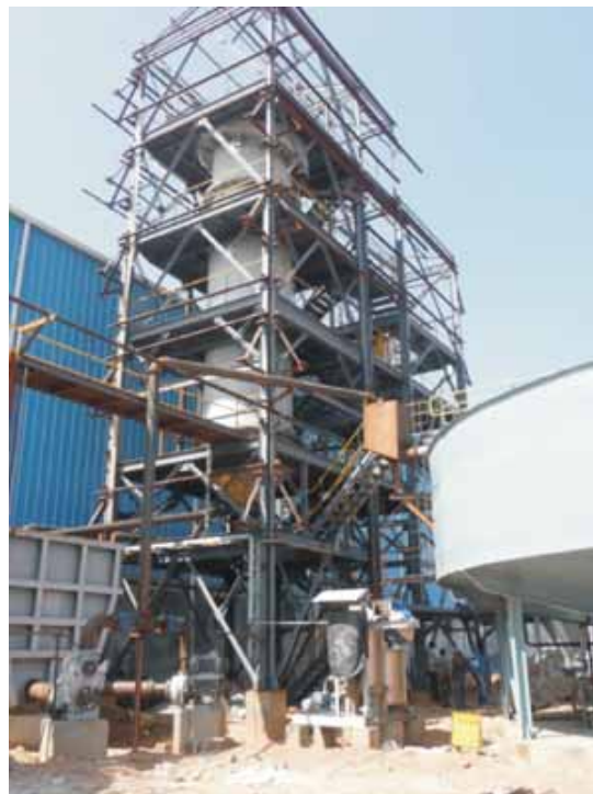
Flotation Column (2.5m dia) erection work in progress at Andhra Baryte Corporation Pvt Ltd, Mangampeta, A.P. for the beneficiation of low grade barytes
